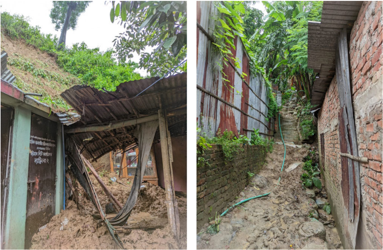
Fig. 8 Landslide disasters occurred on 18 June 2022, killing two people in an urbanised hilly area in Chittagong metropolitan area. Source Fieldwork, the authors
