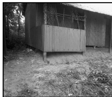
Fig 5: Housing deteriorating due to sandy soil in Shalhati
