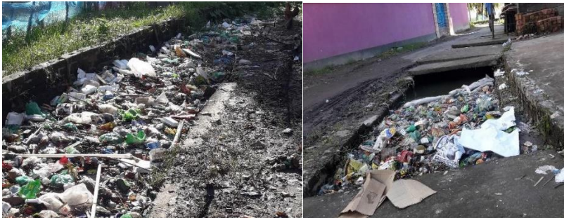
Figure 03: Waste disposal into the drain in front Laboratory School, Teligati, Khulna
