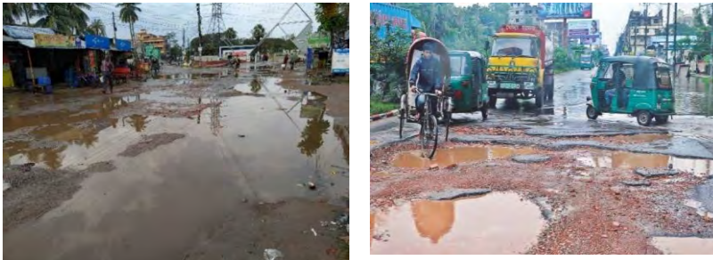
Figure 10 Damage of road due to waterlogging.
