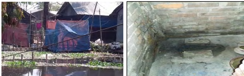
Figure 4: Poor and unhygienic latrine condition at the study area. Source: Author, 2019
