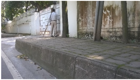
(a) Improper height of footpaths in Gulshan
