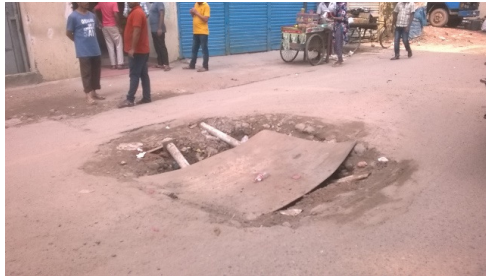
(c) Heavy vehicles destroyed the road surface in Khilkhet.
