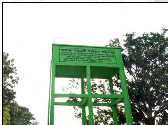
Figure 11 Drinking water tank
